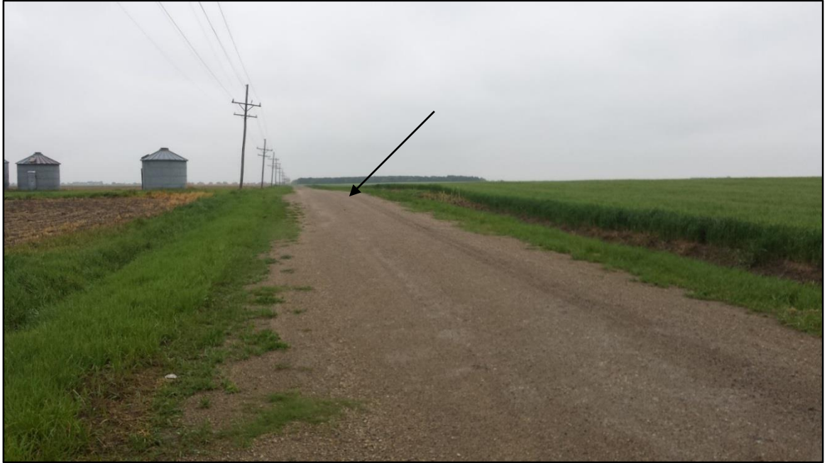
Figure 52. A pressure ridge west of Lost Springs. The ridge runs from the left of the image (north) near the grain silos to the right. It is seen as a slight hump in the road marked by the arrow. Photo taken facing east at: UTM zone 14N – E 669203, N 4268762.
