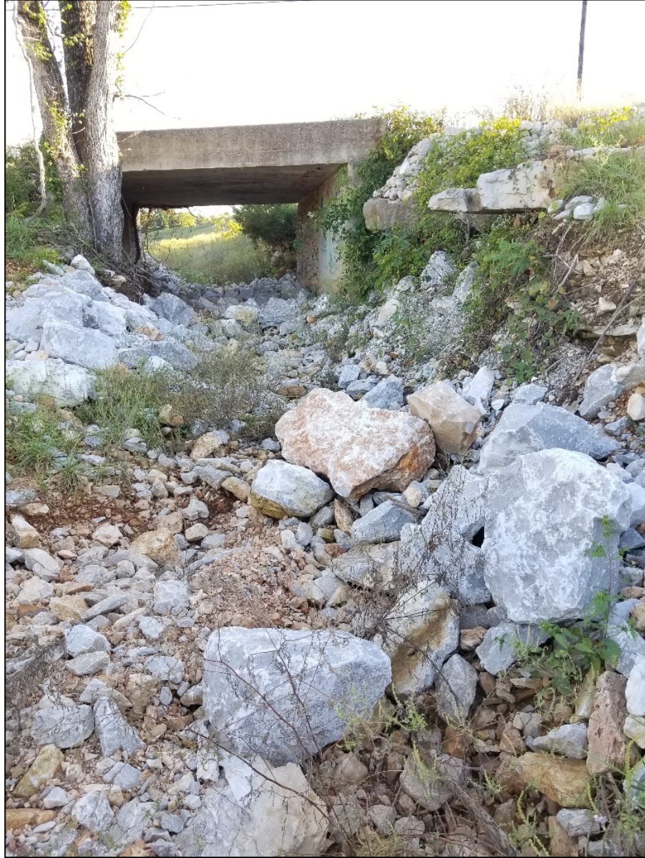
Photograph 6. Road culvert on McKinley Street, location marked on Figure 2. Image is facing north toward the study area. (Photograph taken by Marcia Schulmeister in September 2018).
